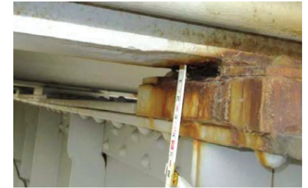
Typical deterioration at steel elements
