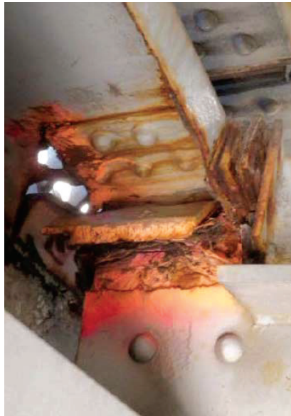
Deterioration at expansion joint support
